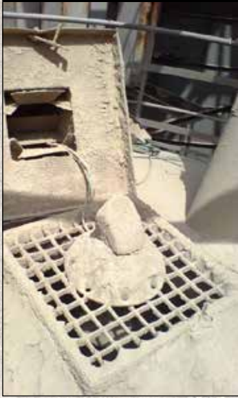
Fully operational sensor on cement silo despite aggressive dust.
